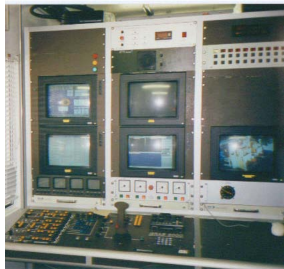
Fig.6 Surface control system
